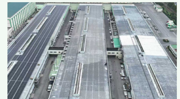
Photovoltaic Project of Henan Anjoy
