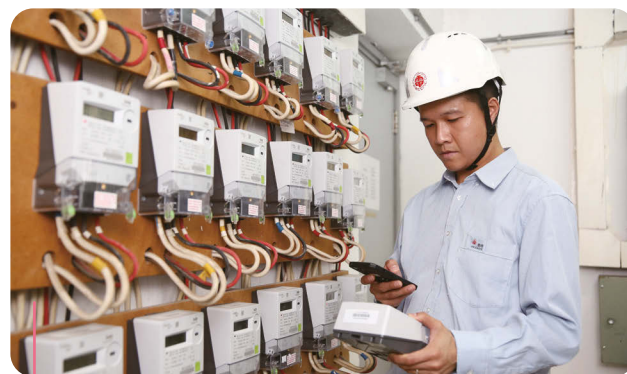
Smart meters and the advanced metering infrastructure not only facilitate better energy management for customers, but also enhance HK Electric's ability for monitoring of the power grid.
