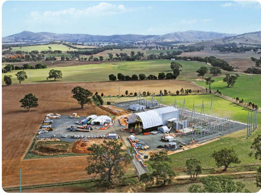
Beon Energy Solutions, VPN's engineering, procurement and construction services arm, constructed Australia's largest synchronous condenser at Ararat Terminal Station, helping stabilise the electricity grid and enable up to 600 MW of new renewable generation in Western Victoria.
