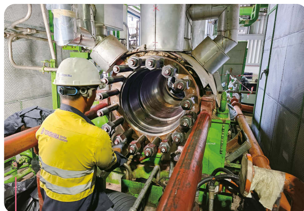
An RPCL mechanic conducts routine inspection and cleaning of the high-pressure boiler feedwater pump casing.
