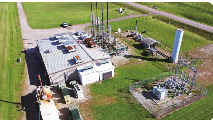
EDL's Brent Run landfill gas power station harnesses methane extracted from the Brent Run landfill near Montrose, Michigan to generate renewable energy.
