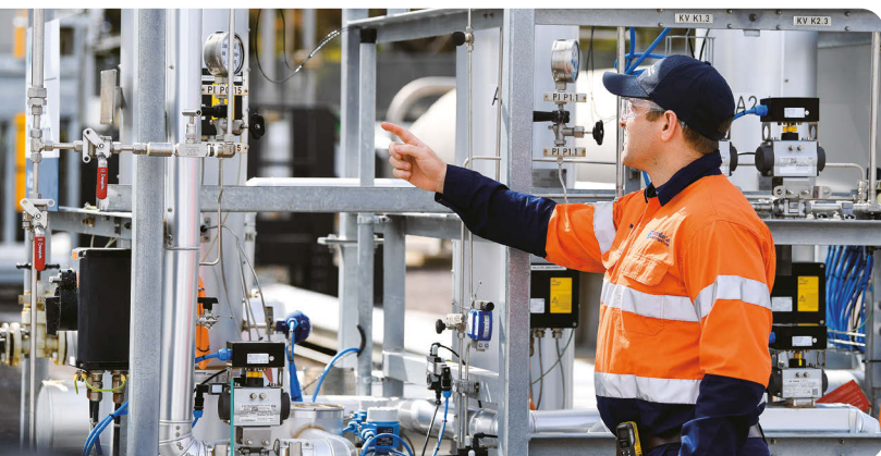
AGN's Hydrogen Park South Australia demonstration project produces renewable hydrogen via electrolysis and blends it into the local gas network.
