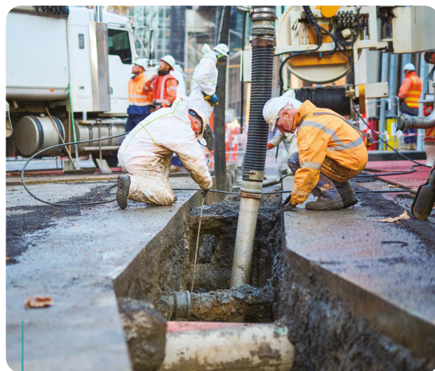
Through the Southbank Jumbo Feeder Project, VPN delivered three new 11kV underground feeders to Melbourne's CBD and Southbank, enhancing network reliability, supporting new customer connections, and enabling upgrade works at the Little Queen Zone Substation.
