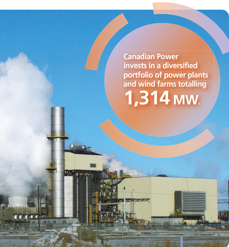
The Meridian combined heat and power plant operated by Canadian Power in Saskatchewan, Canada.
