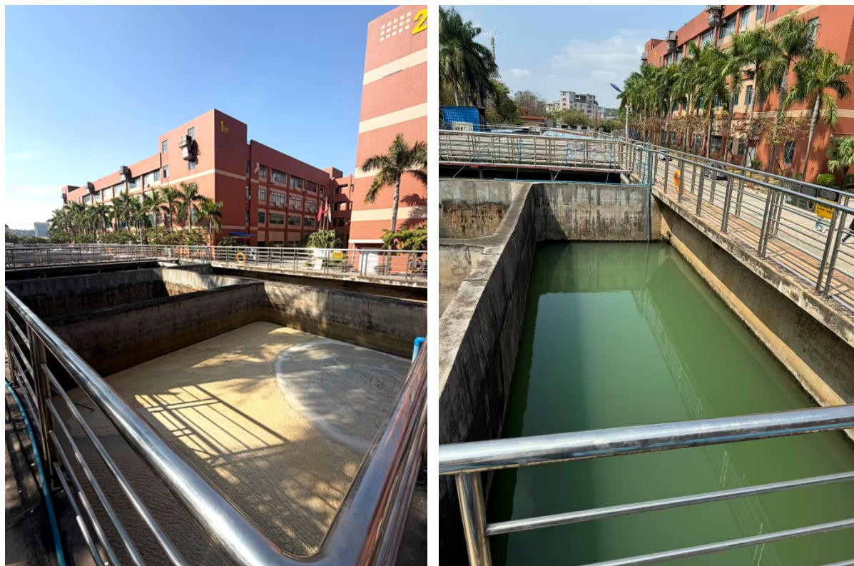
Photo: Onsite wastewater treatment system.
