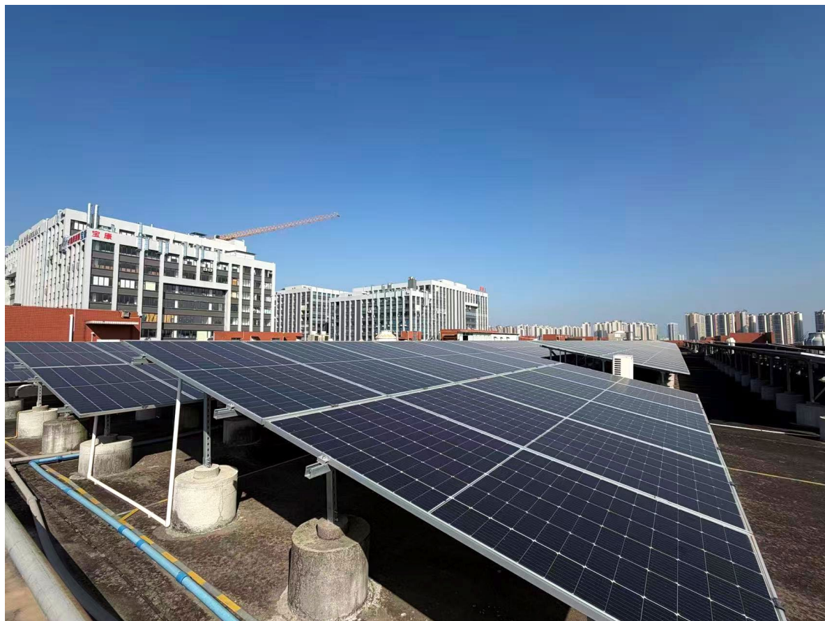
Photo: Rooftop photovoltaic installations
