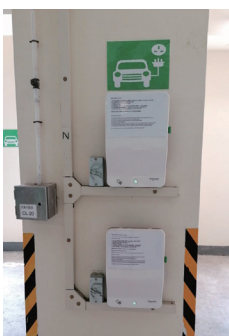
EV Charging Facilities
