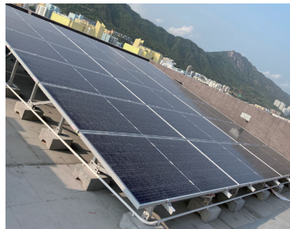
Solar PV System
