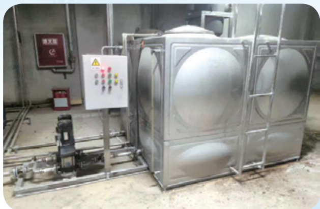
GF water tank
