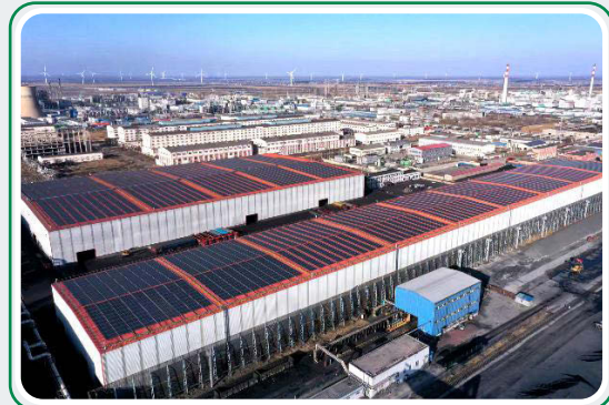
Distributed Photovoltaic Power Station
