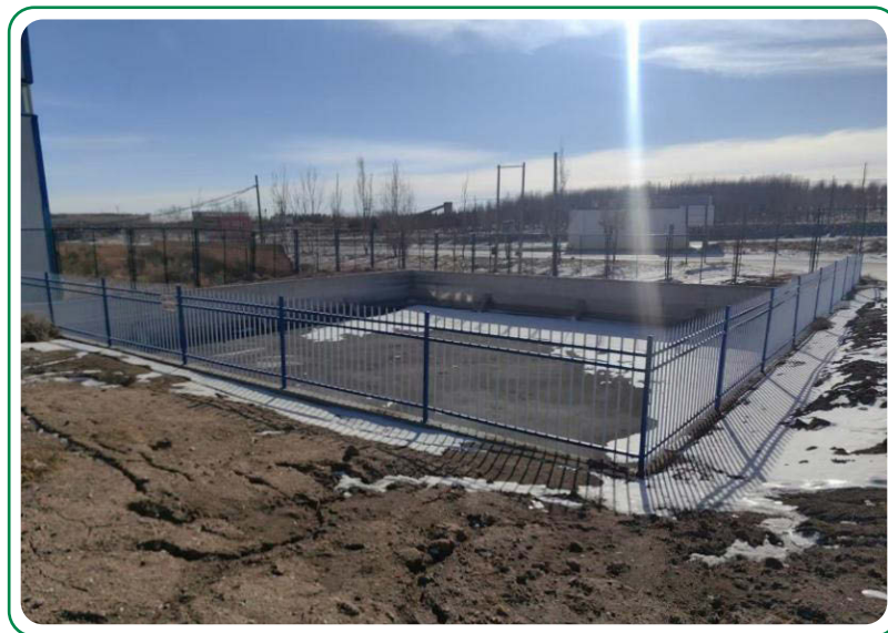
New Rainwater Collection Pool of Baotou-City E-35 Logistics Co., Ltd.
