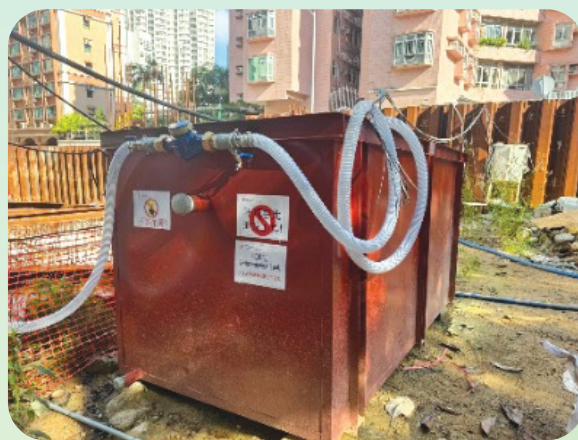
Sedimentation Tank at Construction Site
