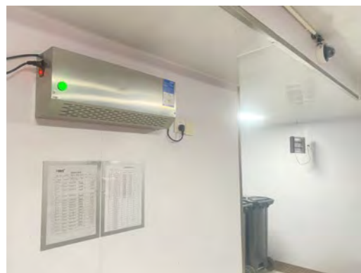
Ozone disinfection and sterilization equipment at waste collection points
